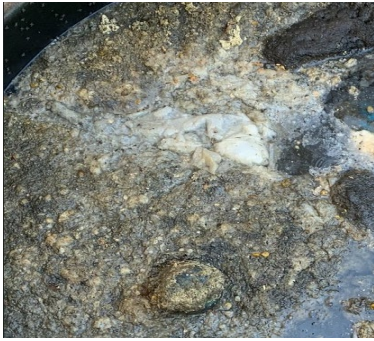
Picture of excess grease and wipes stuck inside a customer's grinder pump.
