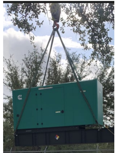
Picture of the generator being delivered by crane at the water plant. During power outages, the generator will automatically turn on to continue to service homes with water from the ground storage tanks.
