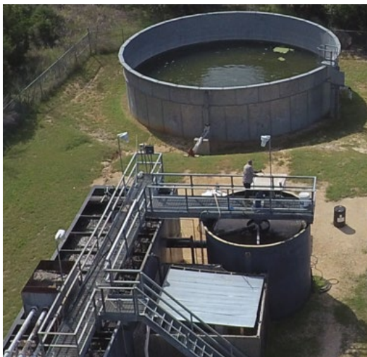
Picture of the wastewater plant that was recently rehabbed. There are now two functioning plants in the event one goes down.
